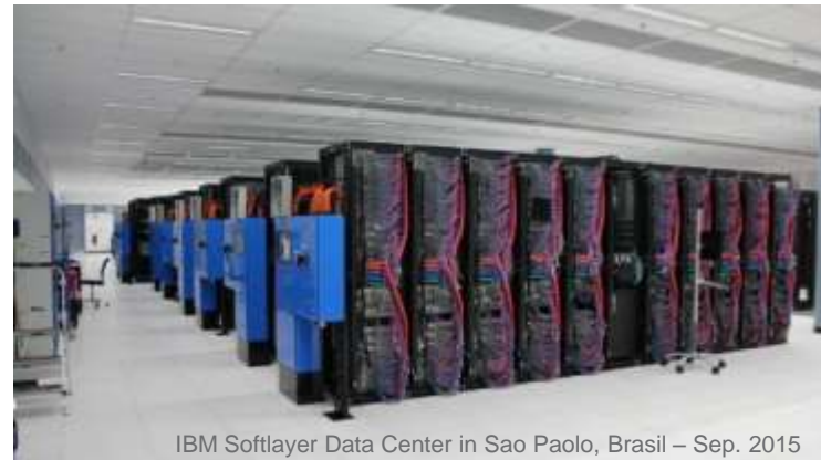
IBM Softlayer Data Center in Sao Paulo, Brasil – Sep. 2015
