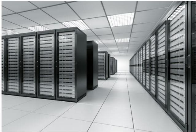
Figure 1: Rows of cabinets full of computer servers in a data center.
